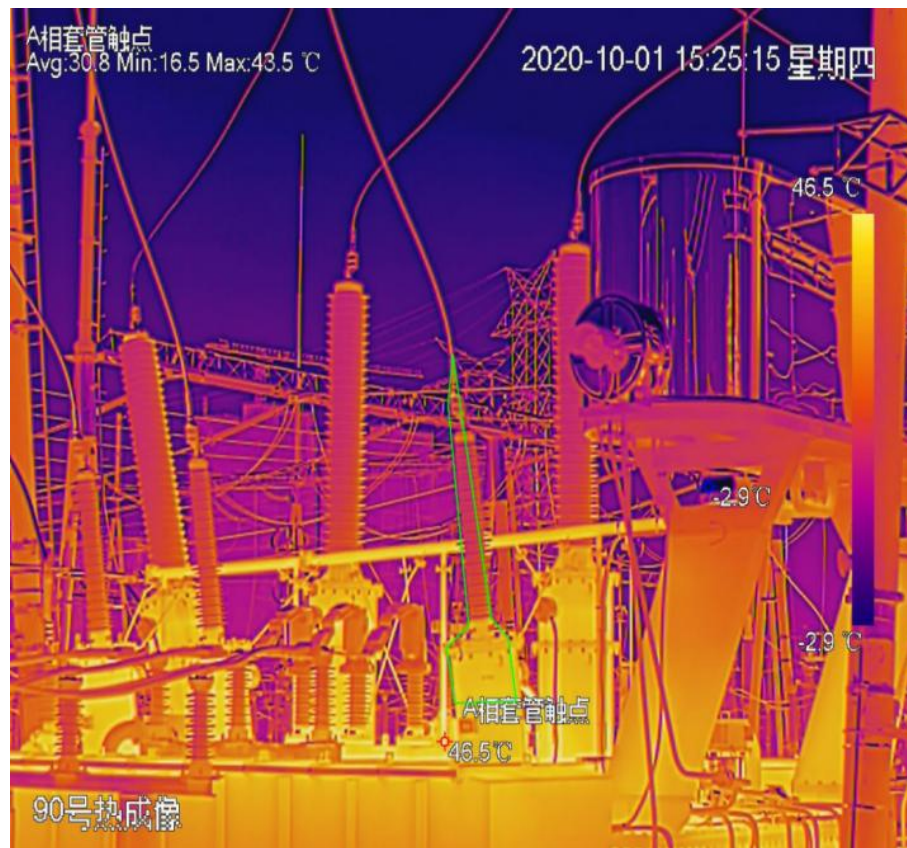
Figure 4 Thermal imaging of phase a contact at 220 kV side bushing on October 1, 2020.
